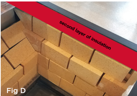
The space blocked in red represents the long skinny strip of insulation described in step 6 above. This second layer of insulation should pack snugly between the top arch rail and the top brick layer. Do the same thing on the left side of the firebox.
